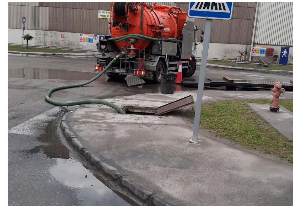
Image 1. Wasted water is refilled to a tanker truck with own pump from gutter.
